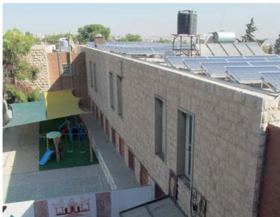
The photovoltaic system saves over €90,000 a year in electricity costs for the TSS.
