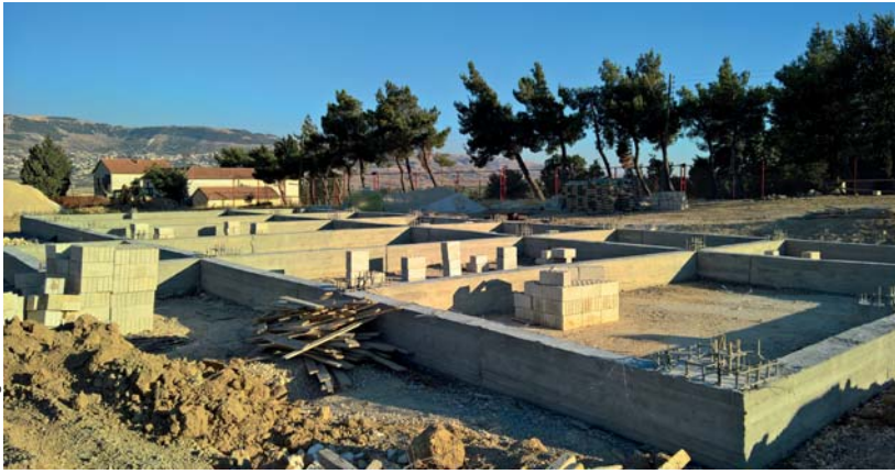
The foundations of the new hall already show how large the new carpentry building will eventually be.
