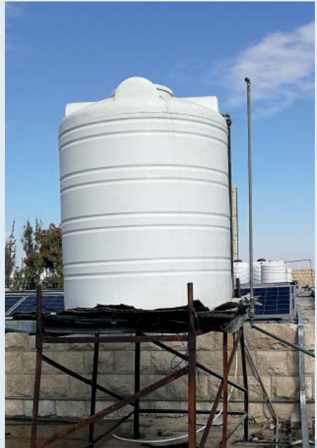
At present, the water tanks on the roof are refilled with water from tanker lorries.
